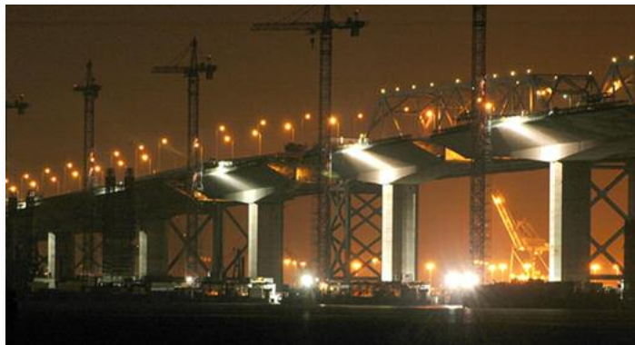
“Night Construction of the Bay Bridge” by Greg Wilson of Berkeley Camera Club Winner: Journalism A Projected Images
